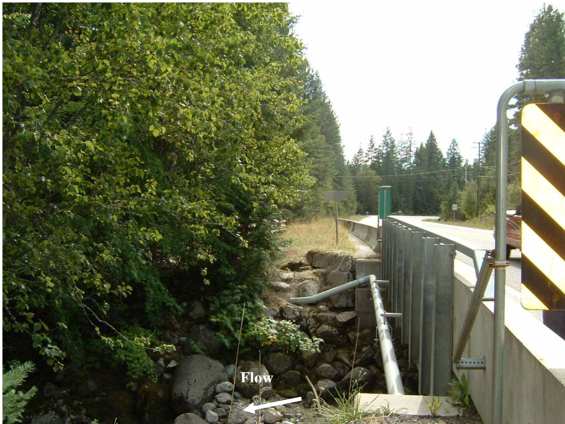
Photo 5 Terasen Gas pipeline on the downstream superstructure of Highway 3A bridge (August 28, 2007)
